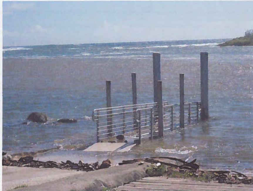
Figure 2: Damaged Boat Ramp Walkway Submerged during High Tide
