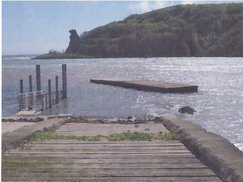
Figure 3: Boat Ramp Facility: Damaged Walkway and Detached Platform Free-floating in Agfayan Bay
